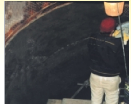
Raw meal duct in a cement plant.
